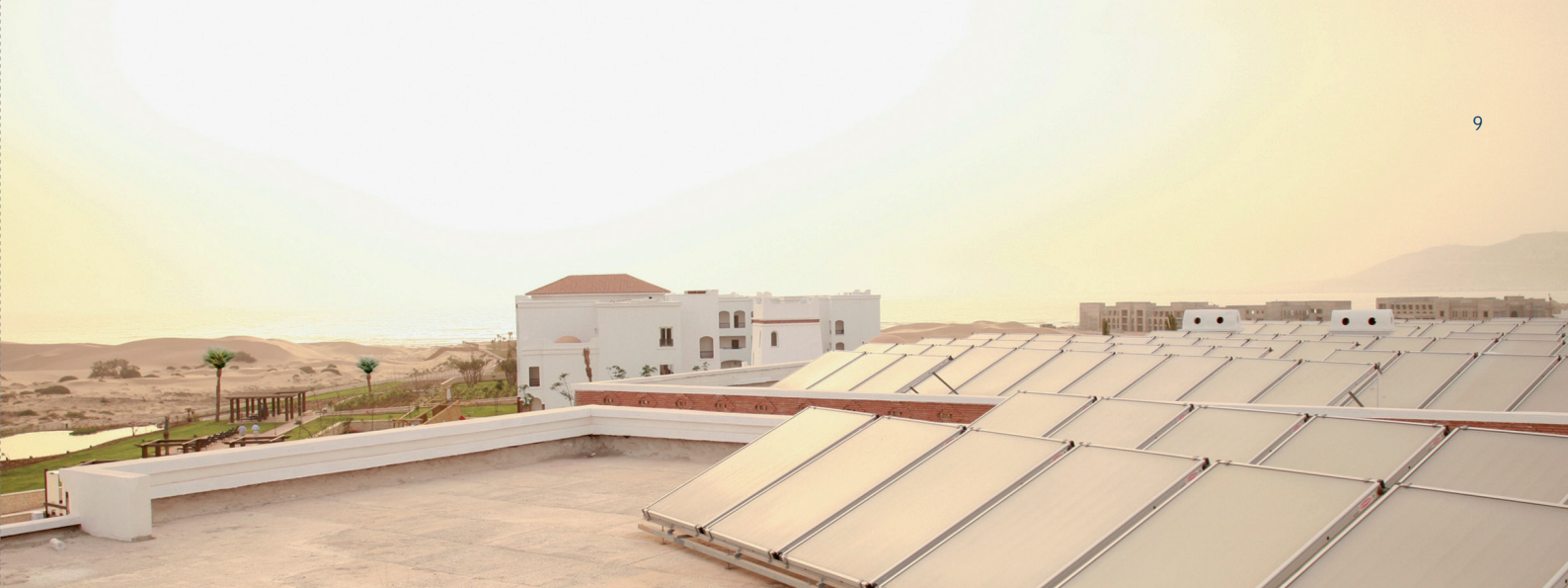
Solar roof on Robinson Club Agadir/Morocco
